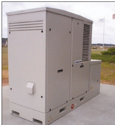
Fuel cell located at Flint Energies in Warner Robins.
